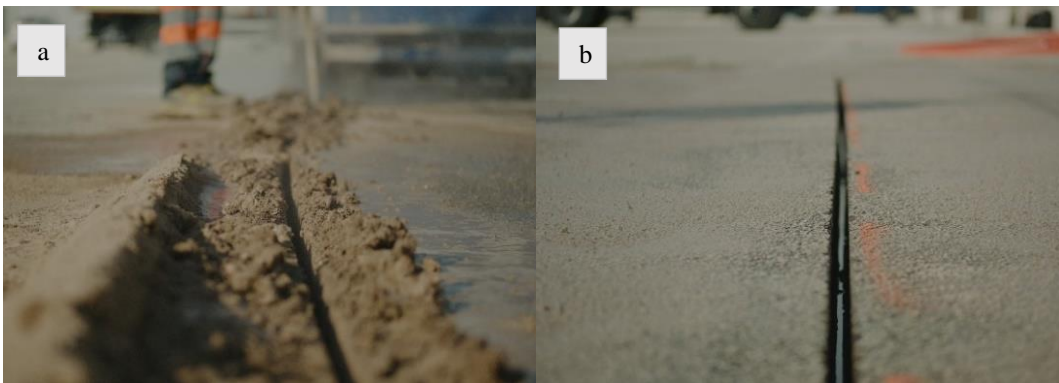
Figure 2. Waste material at the side of the micro-trench after sawing (a); view of the straight and clean edges of the micro-trench (b).
